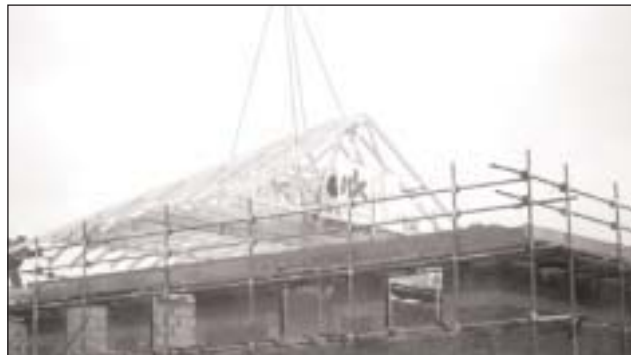
Roof truss built on ground and lifted into position avoiding the need to work over open joisting later on
